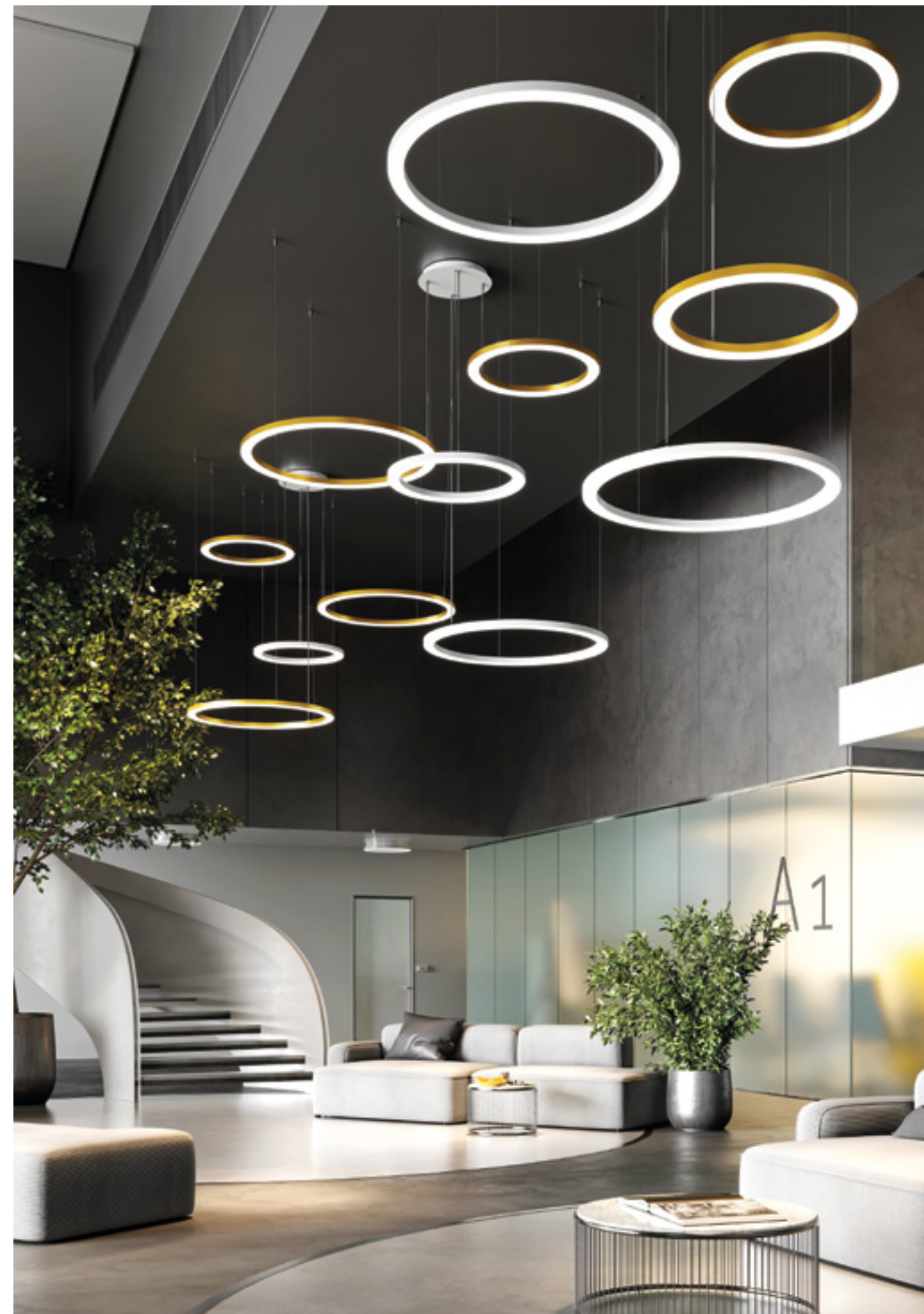
Application of the Solanto Quattro luminaire in an office building lobby.
