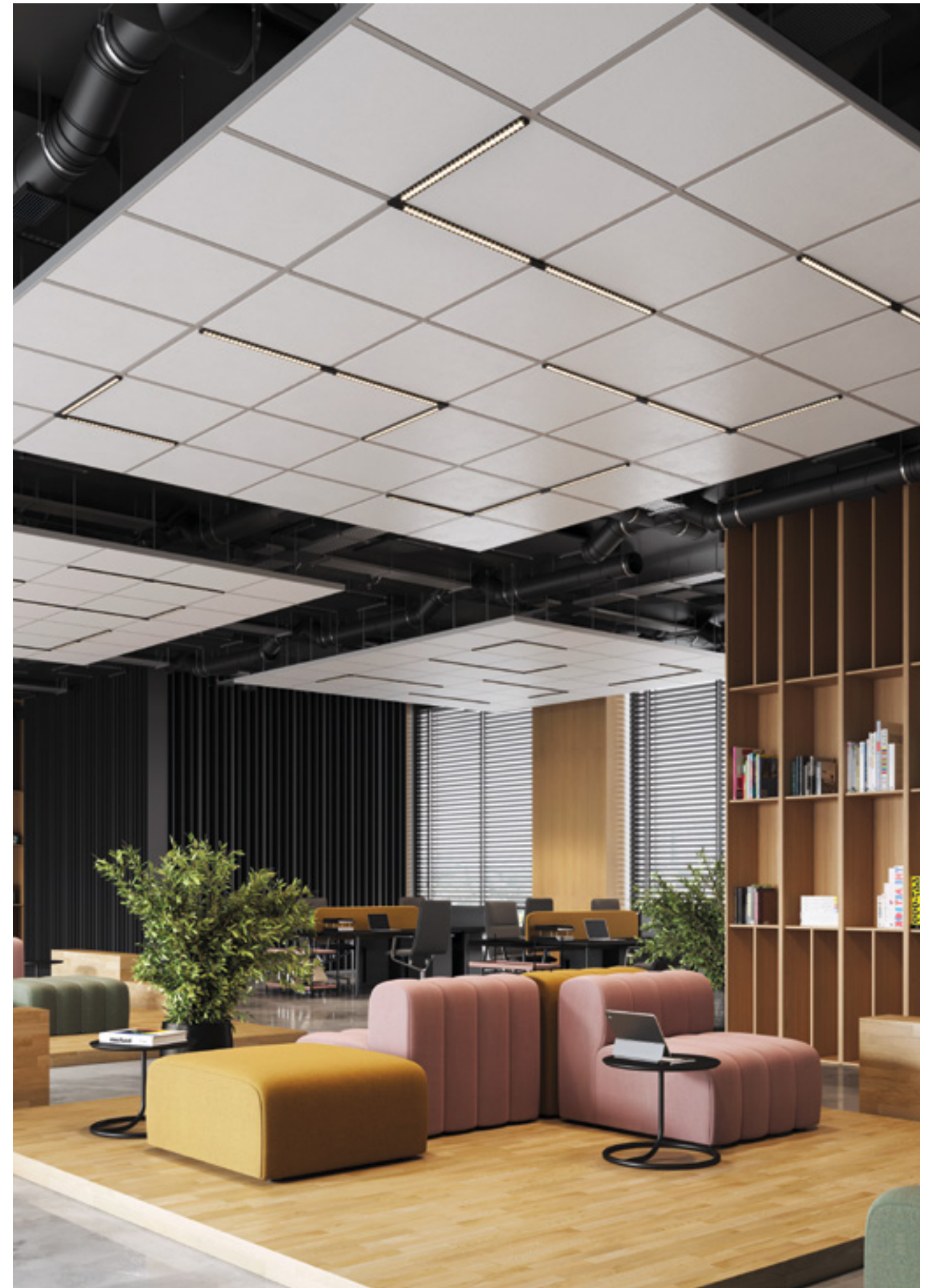
Application of the Terrano system in the office.
