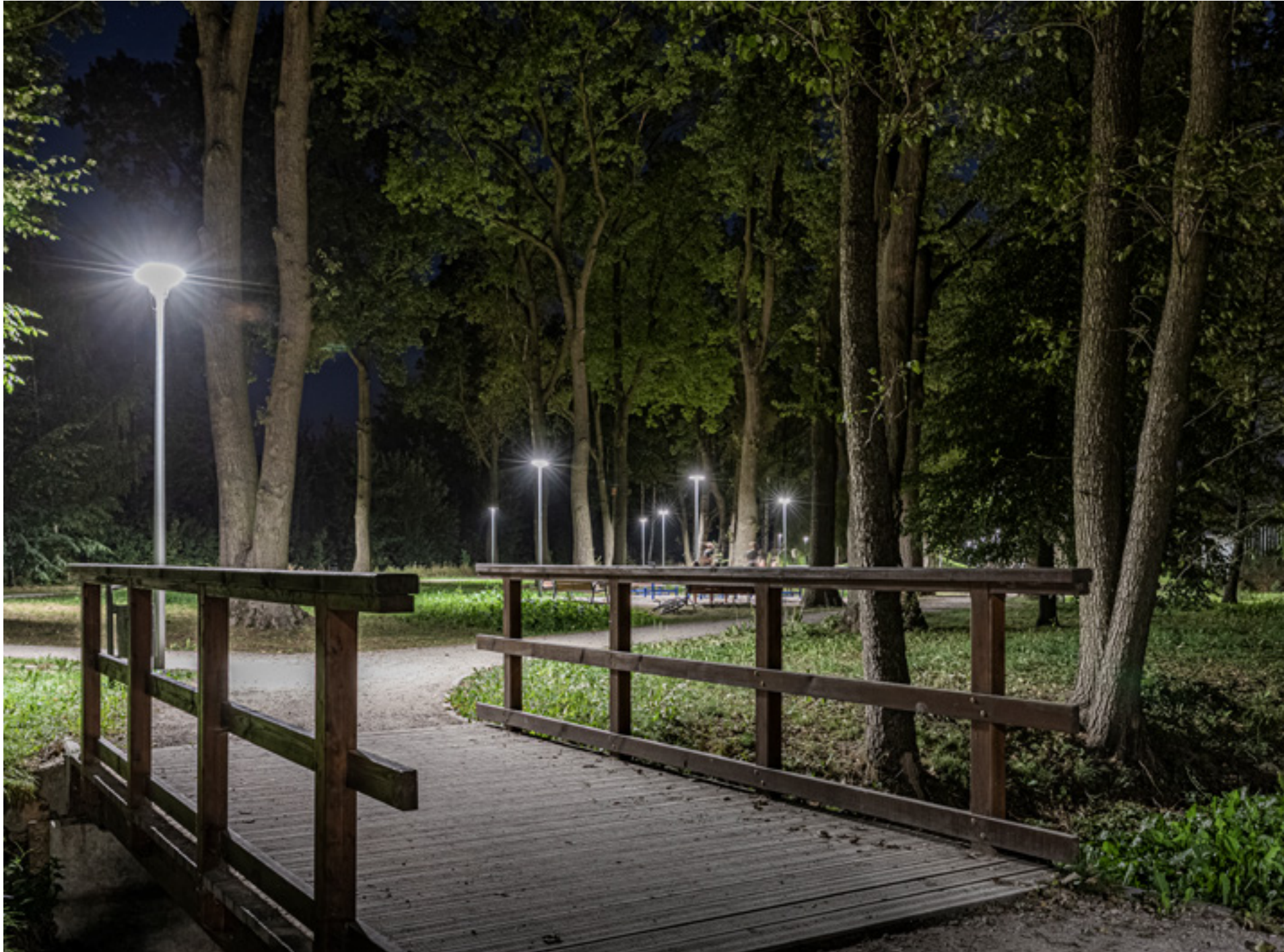
Mitra LED luminaires in the Dębinka park
