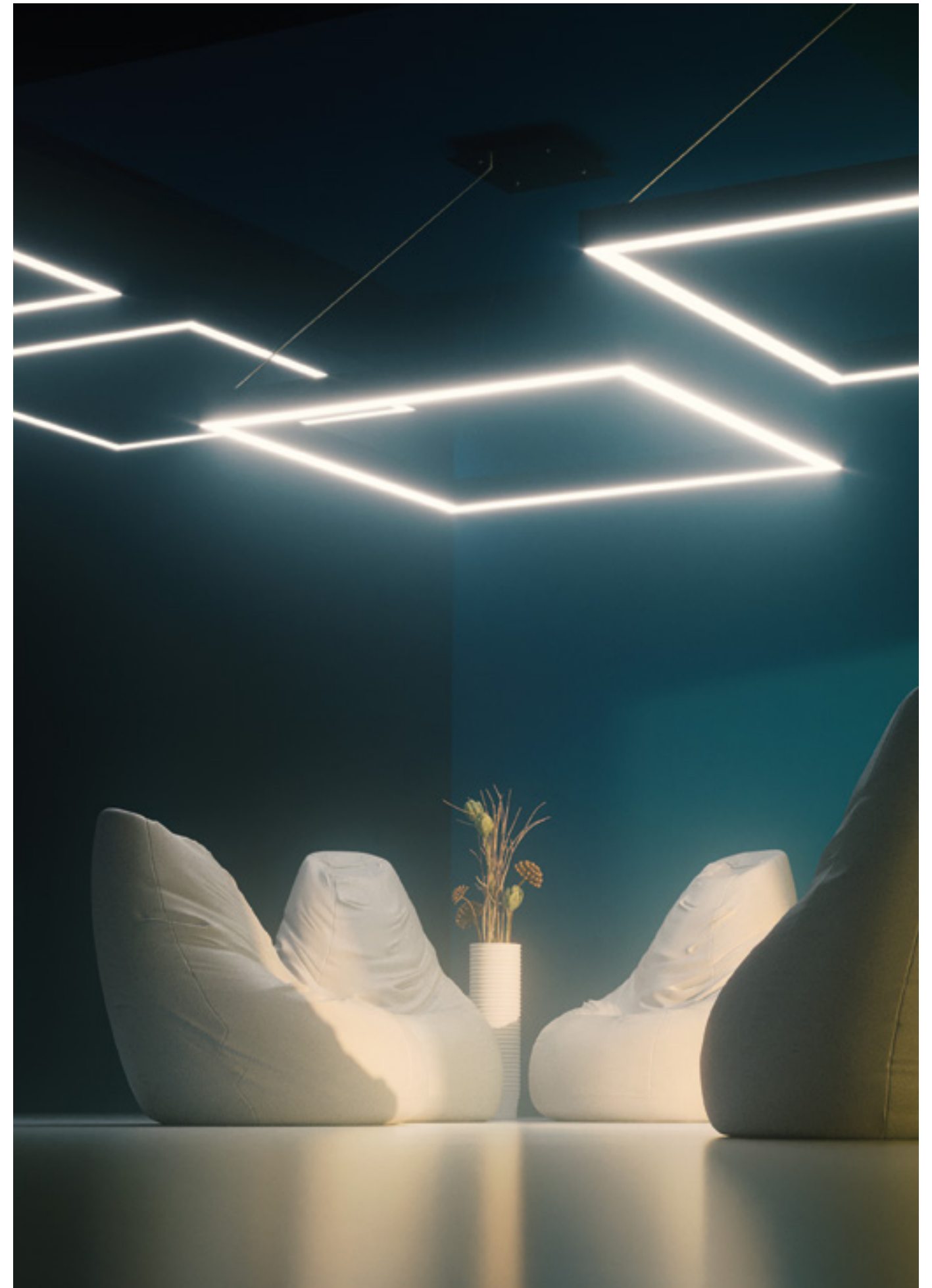
Application the Baris Square 40 LED luminaire.
