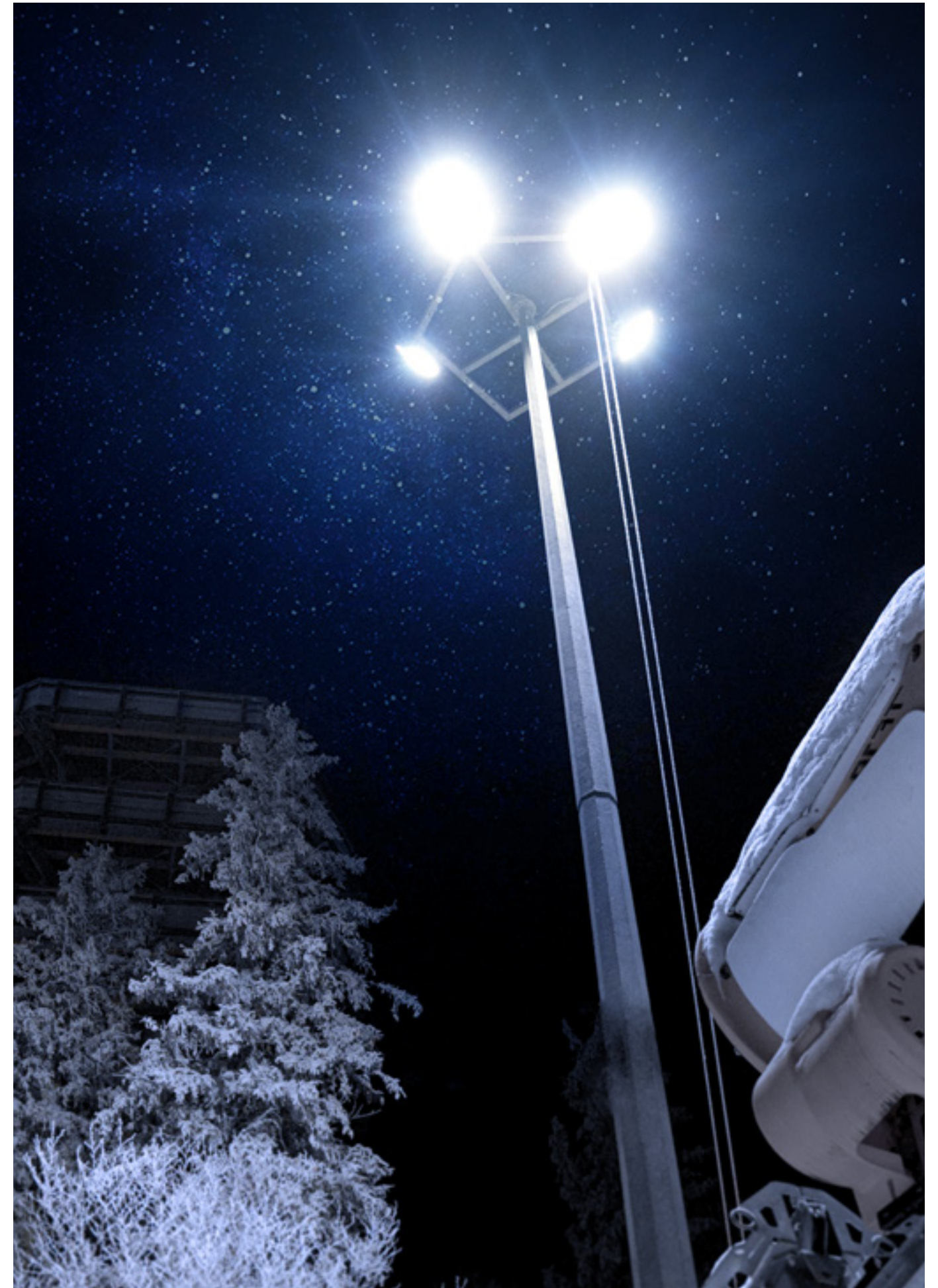
Lighting of the Słotwiny Arena ski slope
