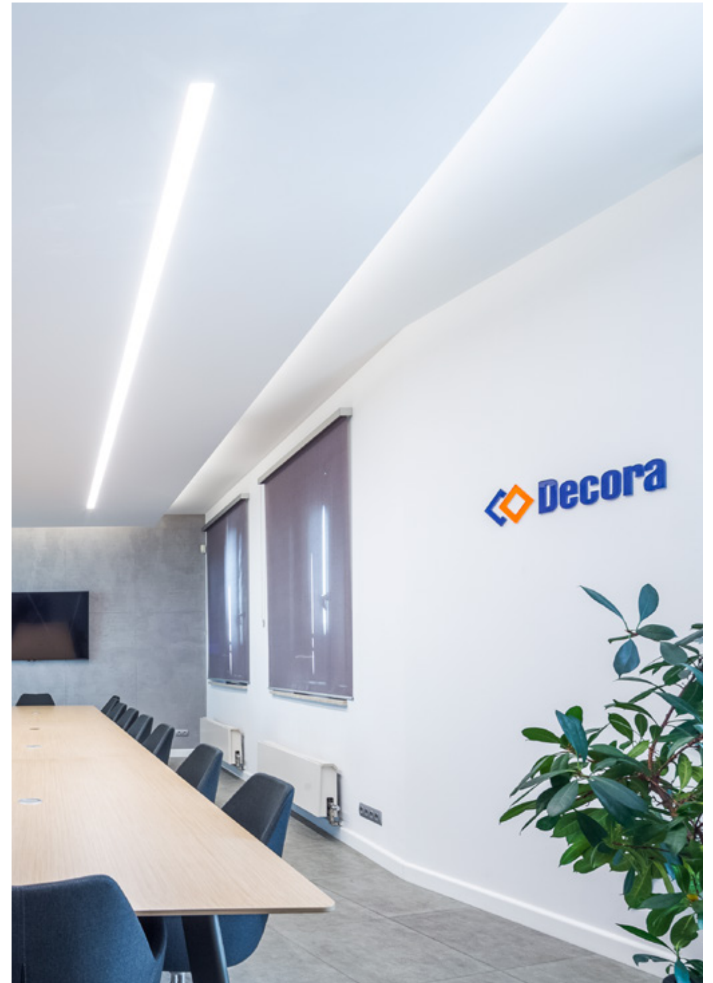
The application of the Elegante LED system in a conference room at Decora S.A. in Środa Wielkopolska.
