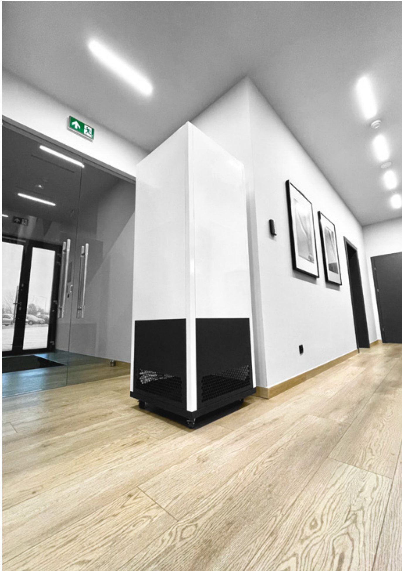
Application of the Sterilon Max Pro UV-C luminaire in the corridor.
